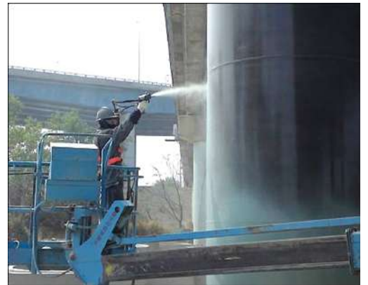
橋墩橋柱鋼構防蝕防護工程 Corrosion resistance polyurea spray coating for steel structure bridges
