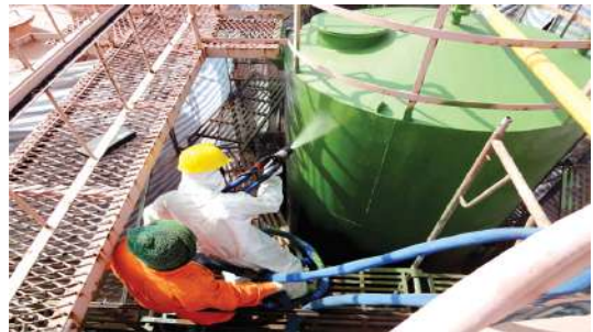
防腐蝕耐候聚脲噴塗 Corrosion and weather resistance - Polyurea spray coating system.
